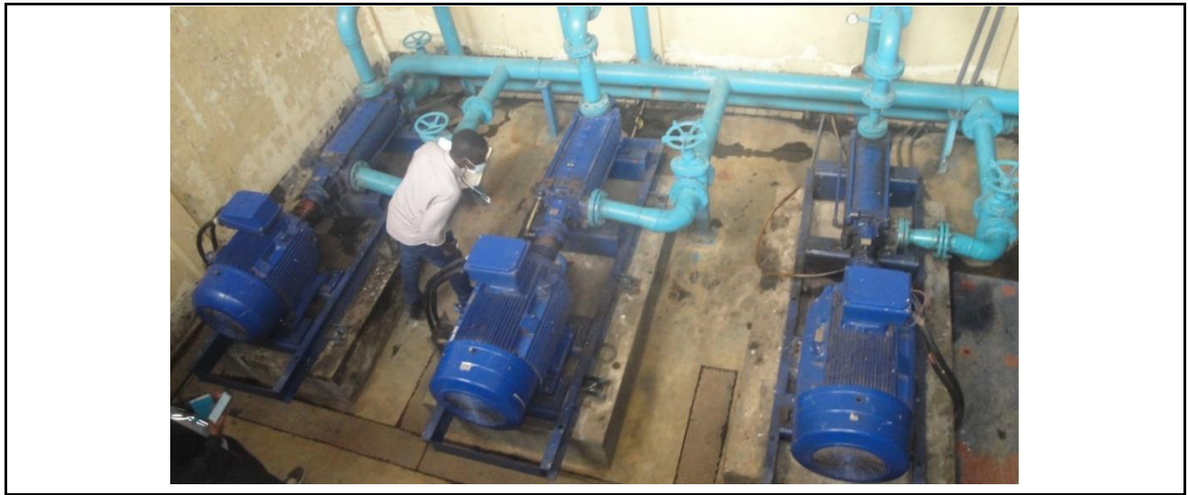
Figure22: Showing Nyamabuye Water Treatment Plant
